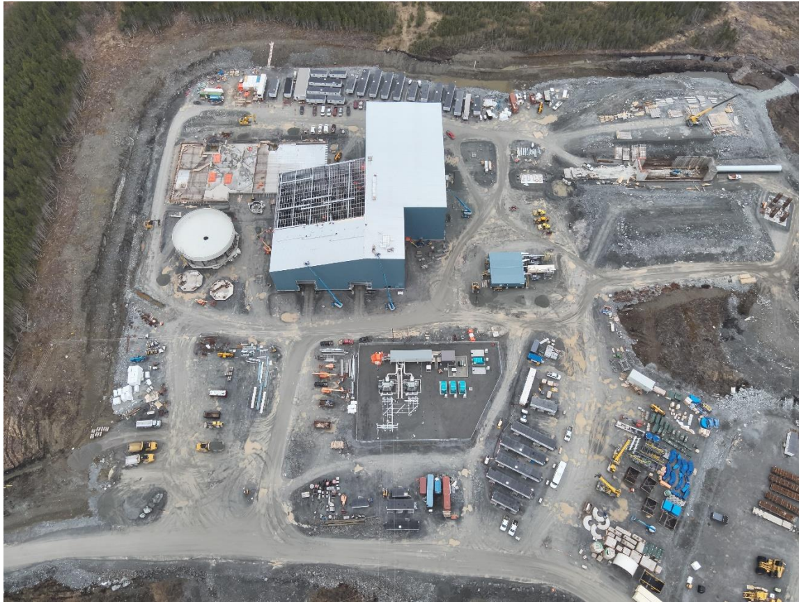
Process Plant East
