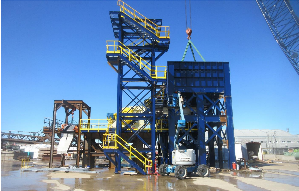
Primary Crushing Plant
