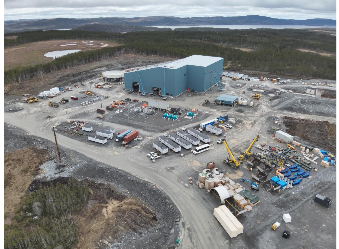
Process Plant Northeast
