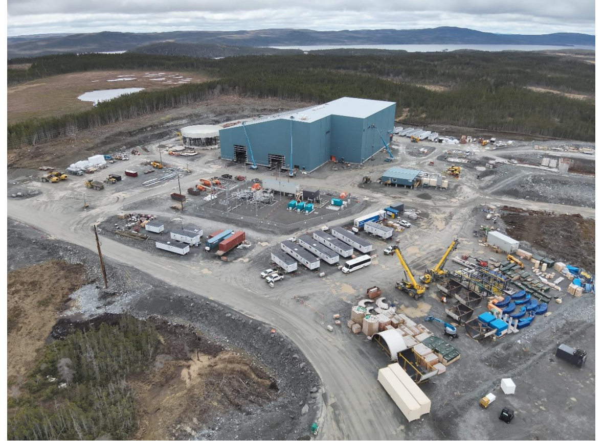
Process Plant Northeast
